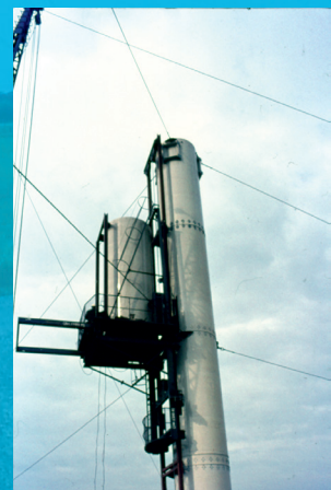
Prefabricated steel cylinders with a diameter of 2 m were mounted on top of each other, until the height of 213 m was reached. At 20 m intervals, three 9.4 m long horizontal booms were mounted on which measuring instruments can be placed. The booms can be swivelled upwards to allow for the replacement of instruments from a higher platform. The mast is guyed at four levels. Photo P.J. Rijkoort, around 1970.
