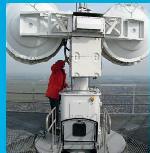
The drizzle surveillance radar IDRA on top of the tower
